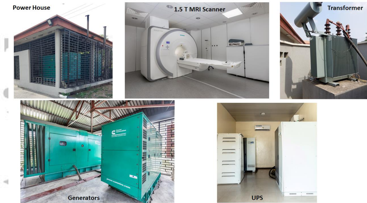
Images of the local energy solution at Crestview Radiology Limited in Lagos, Nigeria for steady power supply for operation of the MRI equipment and other imaging devices.
